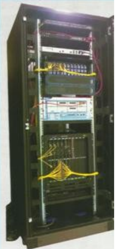
Wired Network Rack Core Switches, Juniper Router, Sonycwal Firewall, Brocade Global Switch etc
